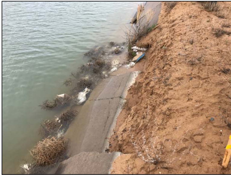
PHOTO: A portion of the deteriorated water canal at the Navajo Indian Irrigation Project negotiation on April 25, 2017.
