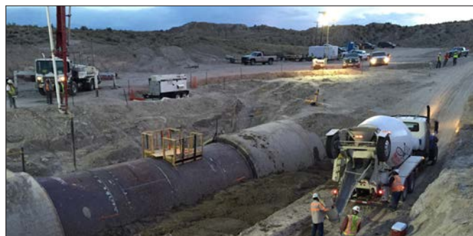
Photo: Workers worked in 24-hour shifts to repair the siphon breach, and was completed on June 10.
