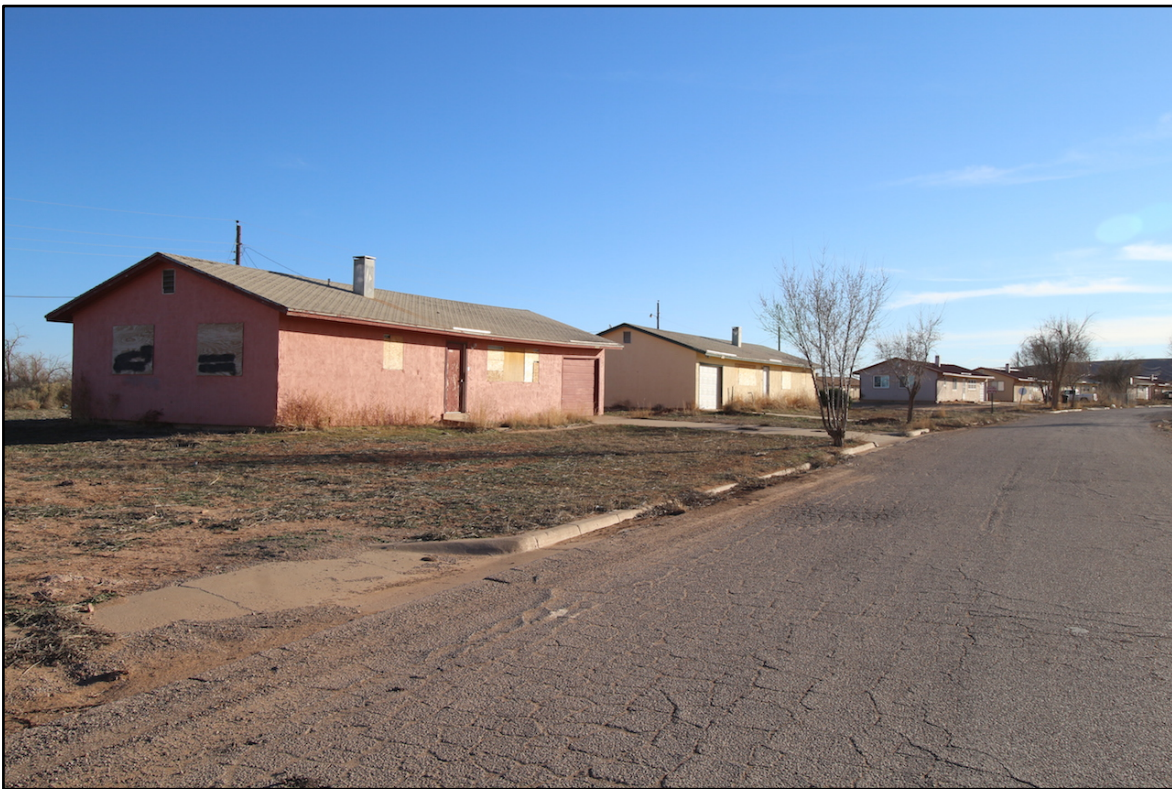
Photo (above): Condemned and unoccupied teacher and staff housing on the Many Farms school campus (2/28/2016).
